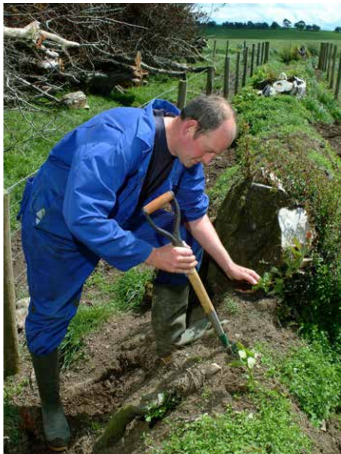
The old hedges were coppiced, gapped up and restored as stockproof boundaries and effective shelter. Photo: Coed Cymru.
